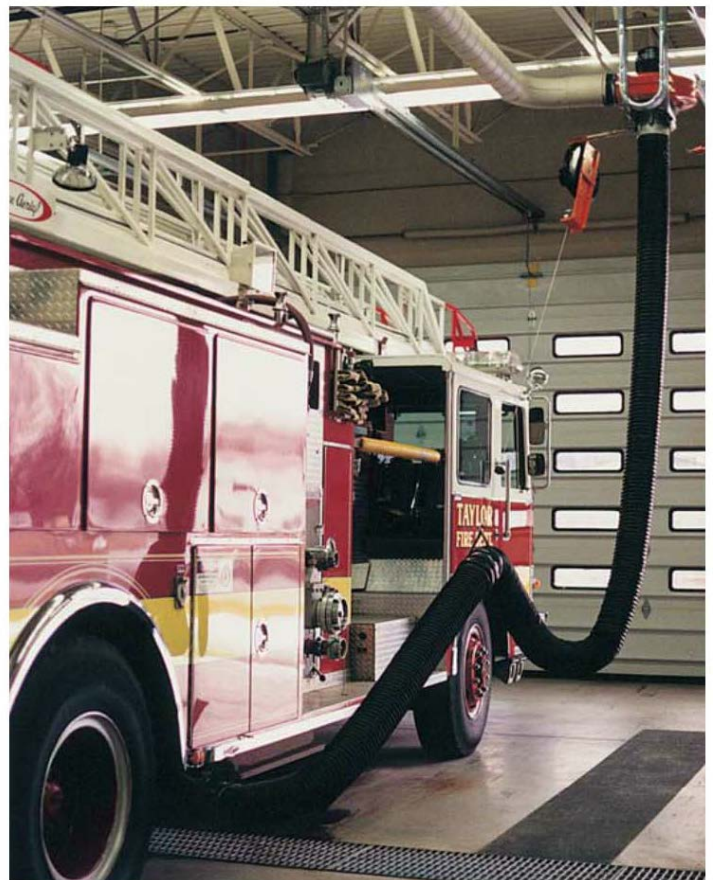
Figure 2-8. Carbon monoxide can quickly build up in a shop, causing asphyxiation and possibly death. Always use exhaust hoses to vent these gases, even if the engine will be running for only a few seconds. (Nederman, Inc.)
